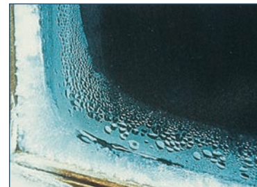
Window condensation can fuel mold growth.
